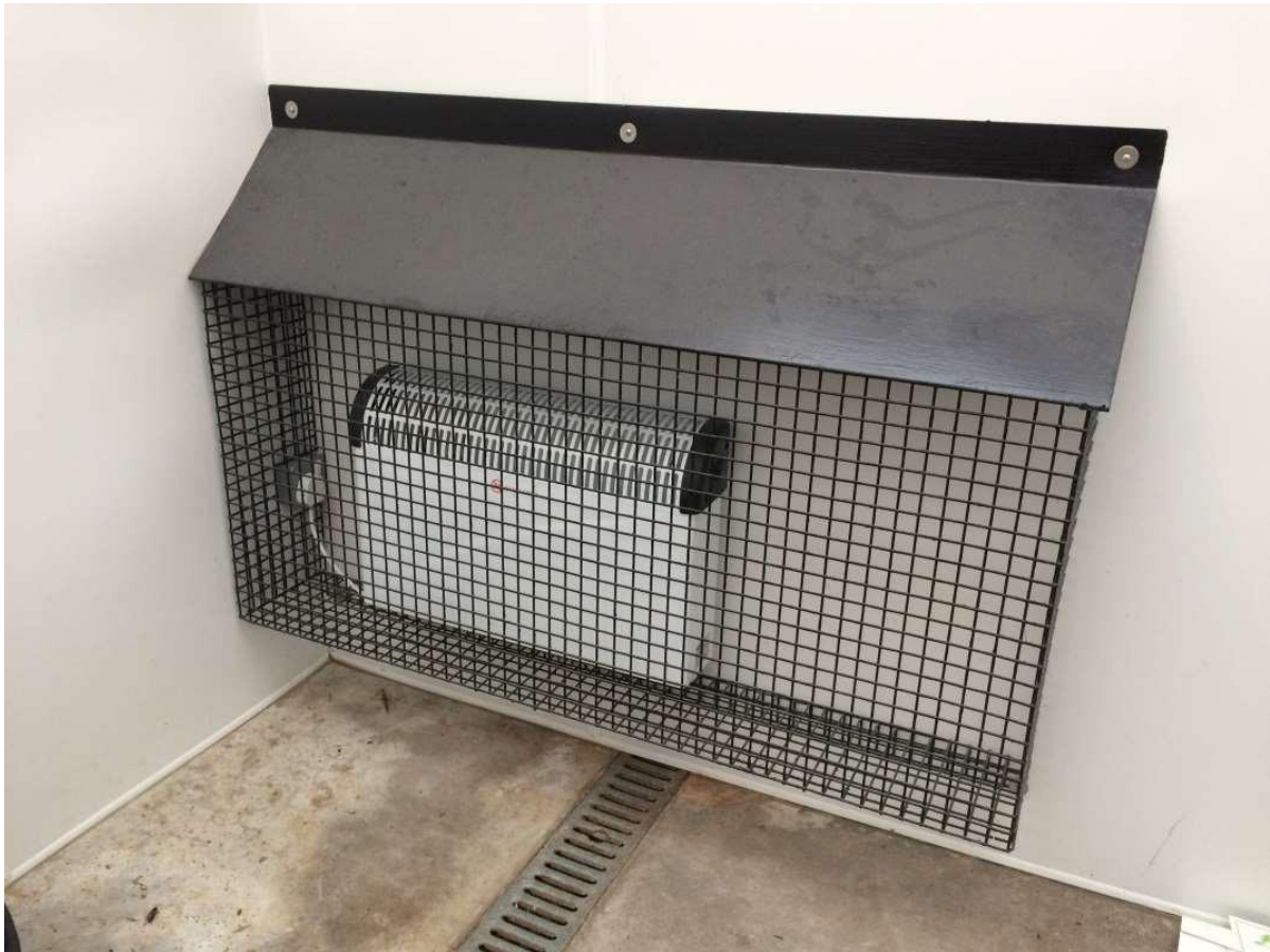
Electric heater with mesh protection and sloping metal cover Chester Zoo
