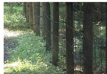
Figure 41: electric cables along the fence © CERZA Zoo
